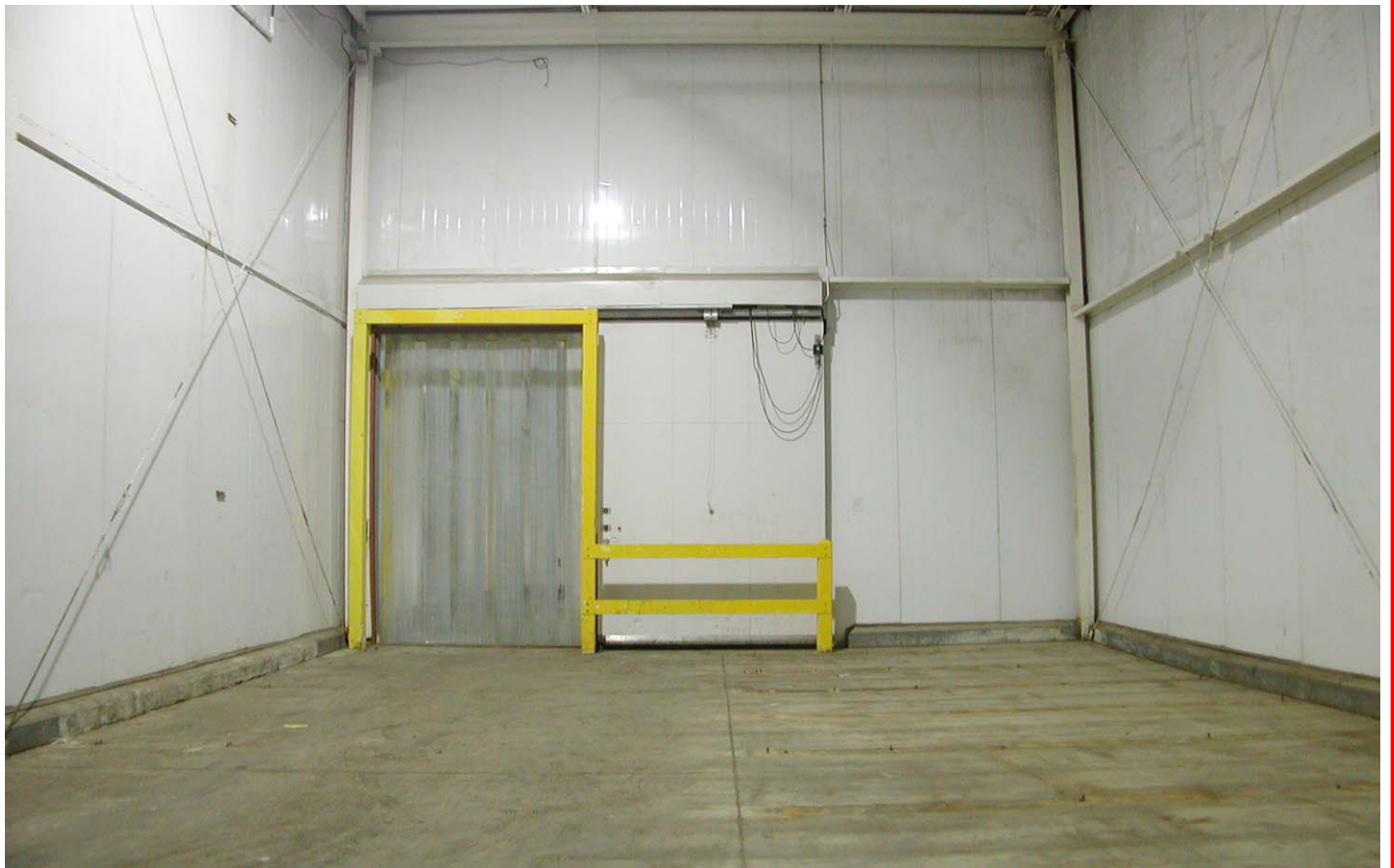
COOLER #3 (CONTROLLED TEMPERATURE 34 DEGREES)
