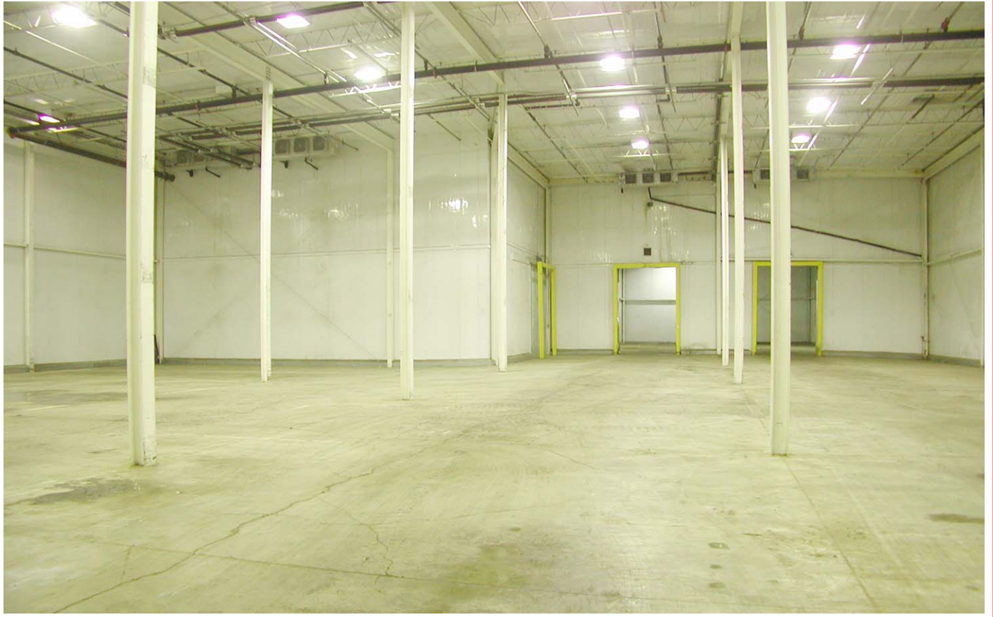
FREEZER (CONTROLLED TEMPERATURE -10 DEGREES)
